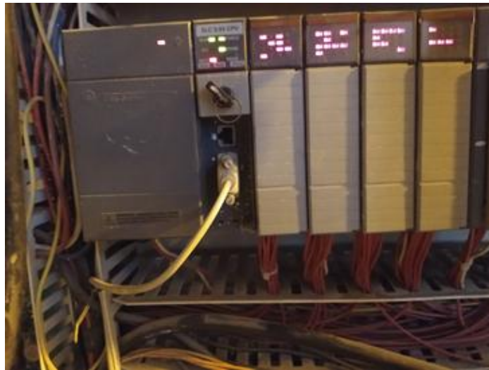
Gambar 7. PLC Limestone Handling
