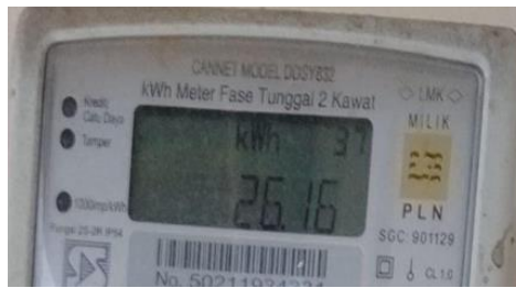
Figure 7. Prepaid kWh Normal Condition
