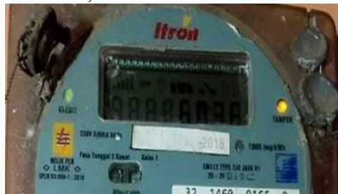
Figure 5. Kwh Meter in Tempering Condition
