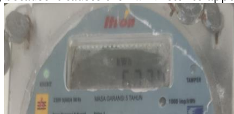
Figure 5. Kwh meter in normal condition
