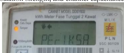
Figure 6. Prepaid kWh Tempering Condition
