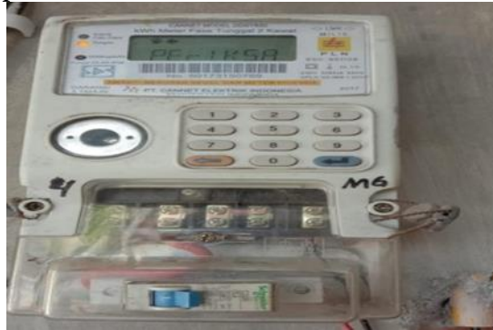
Figure 1. Kwh Meter Cannet
